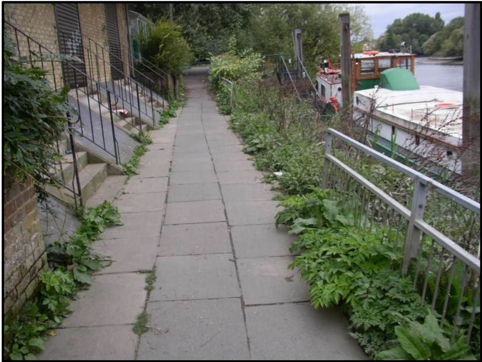
In many places the Edwardian cast iron railings along St Margaret's Riverfront had been replaced with modern galvanised railings in the 1980's but even these had failed in locations as seen here on 17 Sept 2004 as one approaches Isleworth Promenade.
