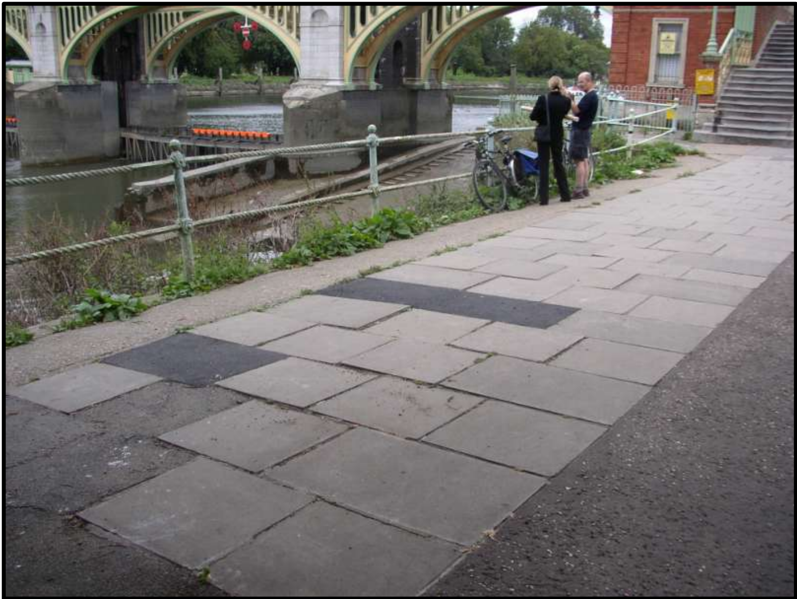
Inspecting the old broken Edwardian cast iron railings along St Margaret's Riverfront 17 Sept 2004 before works started by grade II* Richmond Lock
