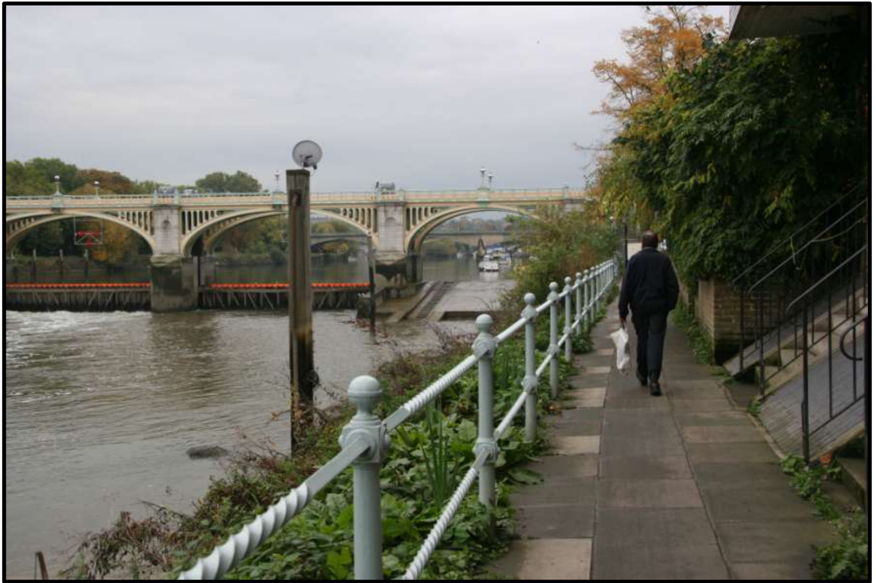
The restored Edwardian cast iron railings along St Margaret's Riverfront and Isleworth Promenade 1 October 2007 looking towards the grade II* Richmond Lock. Nearly a mile of cast iron railings were restored as part of the works.
