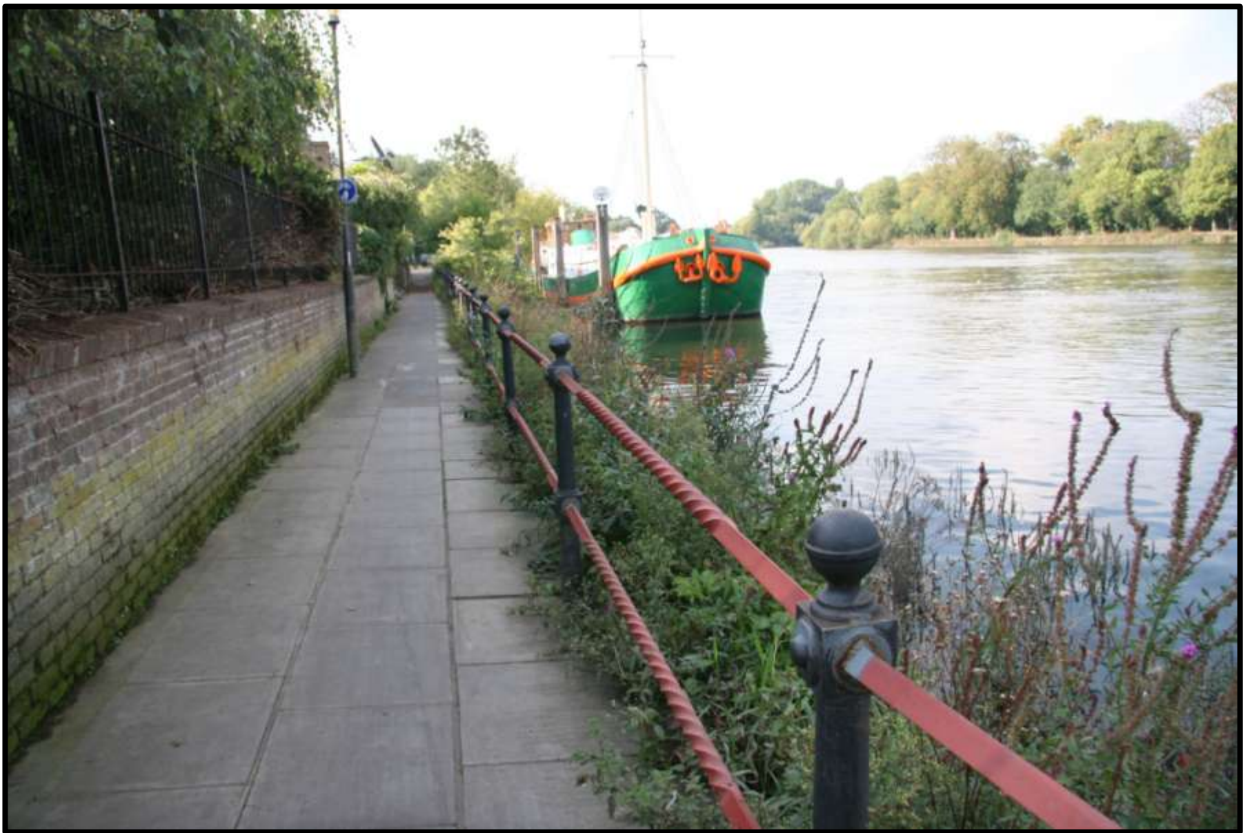
Works underway to restore the Edwardian cast iron railings along St Margaret's Riverfront and Isleworth Promenade 14 September 2007. Nearly a mile of cast iron railings were restored as part of the works.
